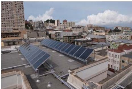
Solar thermal cuts operating costs for commercial buildings that use large amounts of hot water or other fluids.
