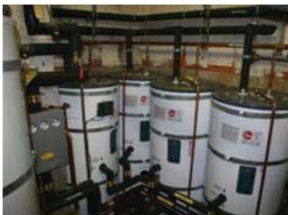
Mechanical room configuration
