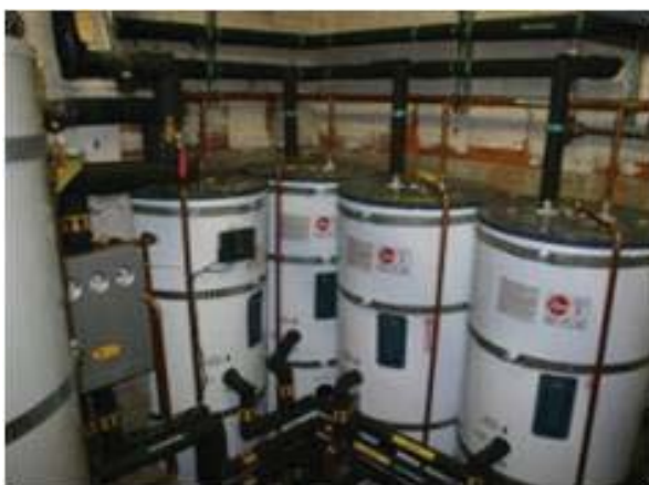
Mechanical room configuration
