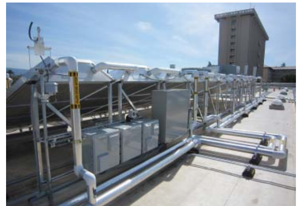
Rear view of MCT collectors & piping at the Benson Center
