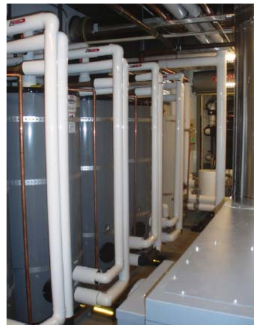
Mechanical room configuration
